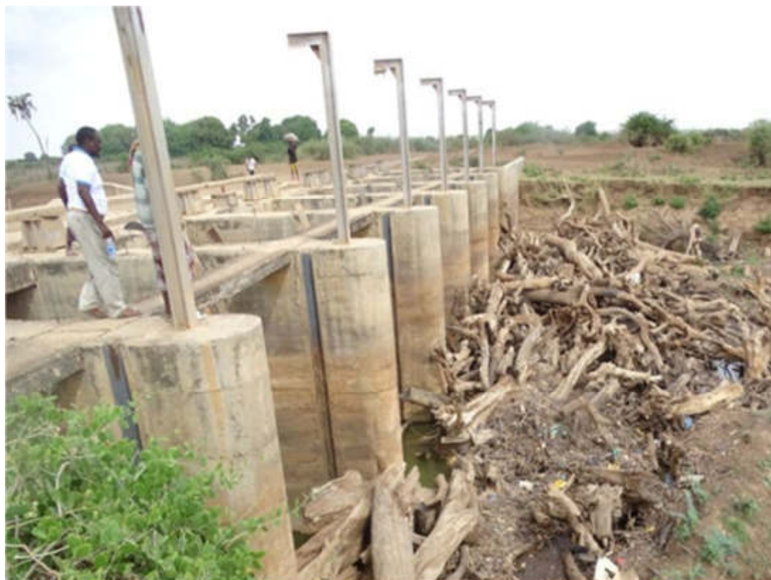
Figure 5.14: Sabuun barrage; without steel gates, water levels are controlled by wooden debris
