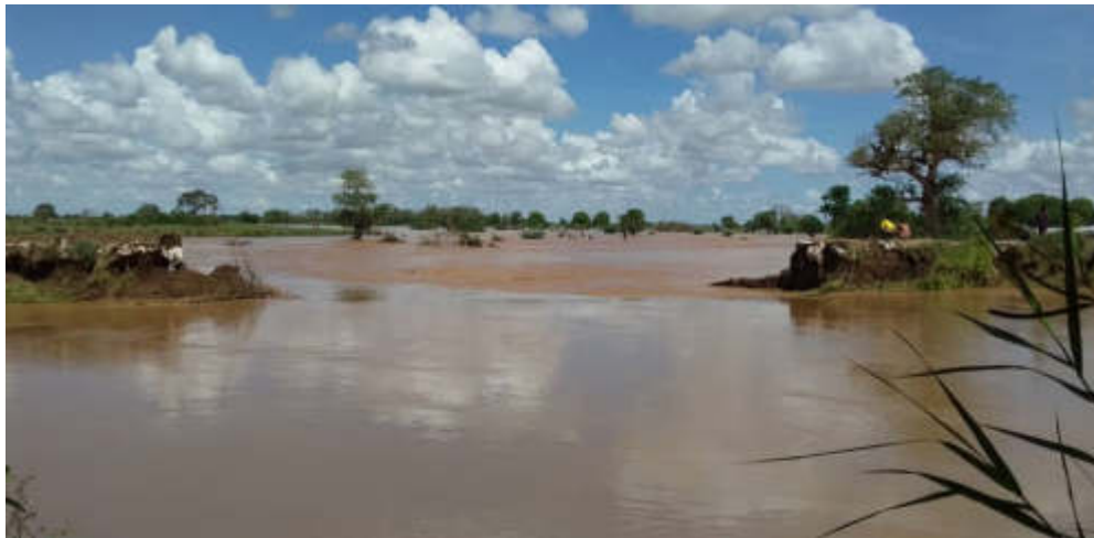
Figure 5.11: Deliberate embankment breach for irrigation purposes
