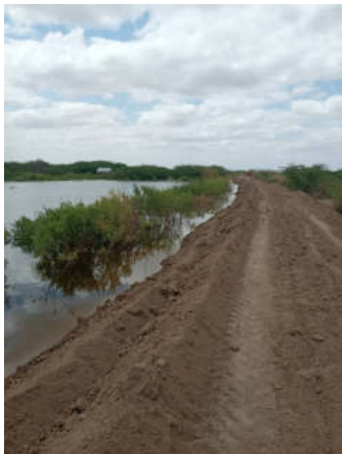
Figure 5.4: Dike (in combination with a road) constructed perpendicular to the Shabelle upstream of Beledweyne
