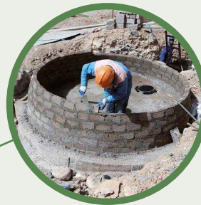
Construction of the fixed-dome type agricultural digester in the village Ait Idir.
